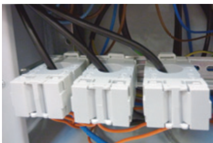
Current transformers for cables mounted on DIN rail
