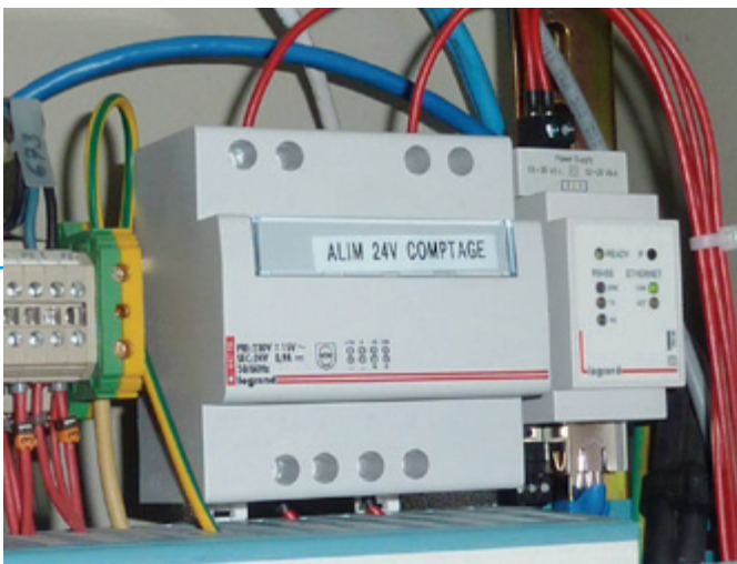
24 V power supply and IP converter
